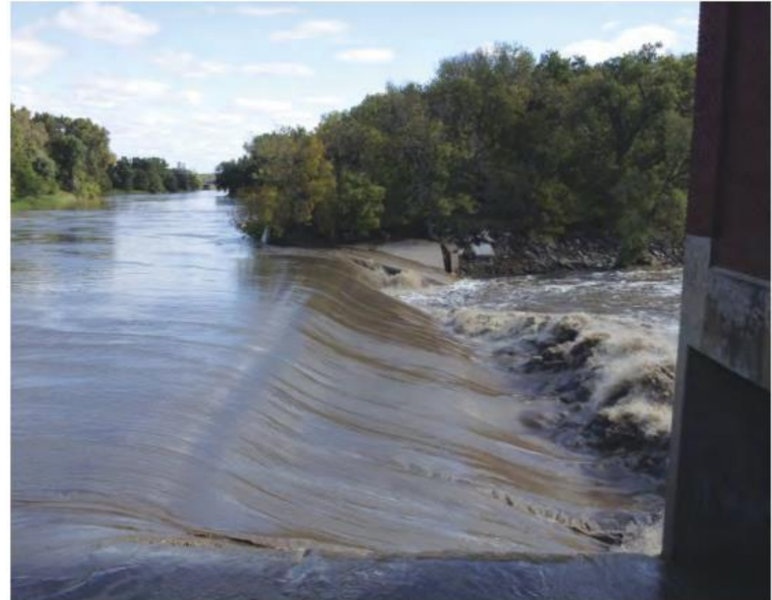
Big Blue River as it appeared on October 3, 2014, with approximately 9,000 c.f.s. spilling over the dam. Erosion of the face of the dam is clearly evident on the far end. Streamflow over the dam on May 4, 2018, when it ultimately failed was approximately 4,000 c.f.s.
