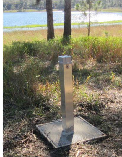
Instruments in the ground monitor indicators of water quality
