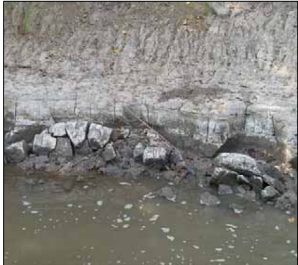
Photograph 5-1. Highly erodible bank on Delaware River with steep slope and no vegetation.
