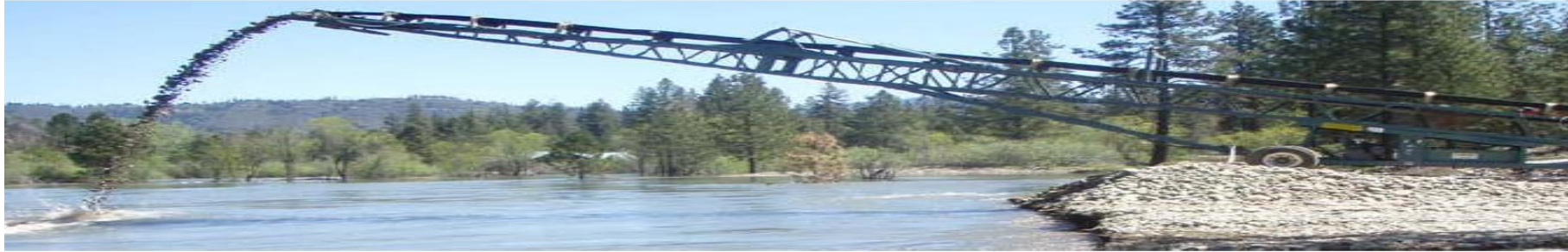
Gravel injection below Lewiston Dam, Trinity River
