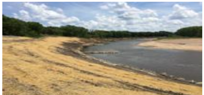
Same site following construction (taken looking back at where the first picture was taken).
